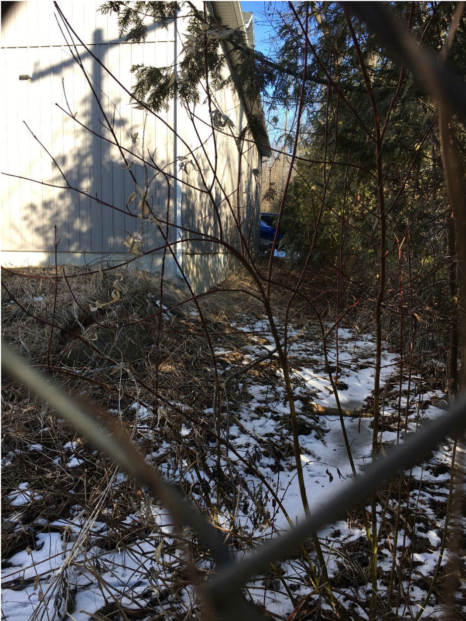
Photo 2: shows the downspouts on the south west corner of the building directing water west, instead of to the rear of the property as indicated by the plan.
