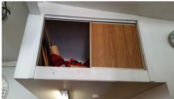
(photo: storage in the garage bay requires ladder access and is limited in storage space and weight limits)
