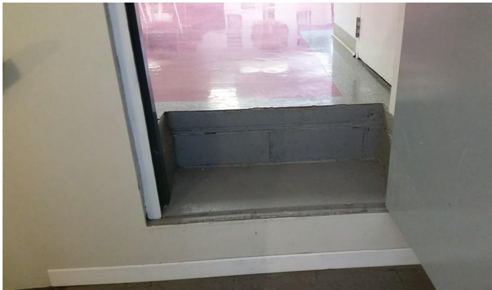
(photo: steps from the second floor Chief's office to the crew/training room)
