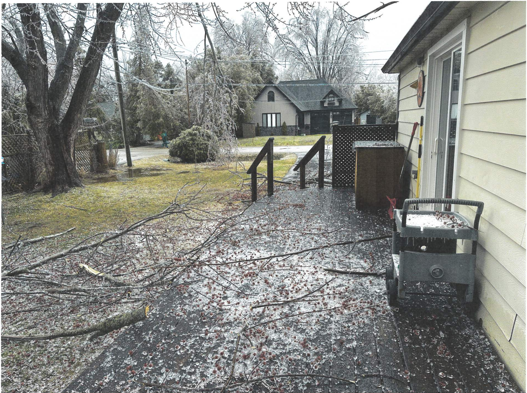
Any storm damage branches we know of from the marked tree fell into our yard on our patio. 4
